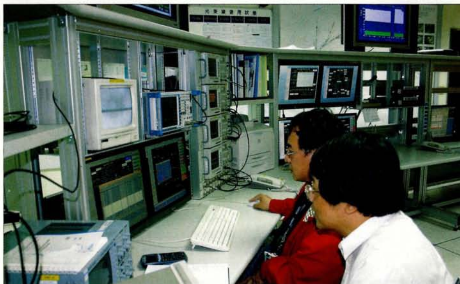
NSRRC's control room with top-up operation displayed on the monitor in the background.
